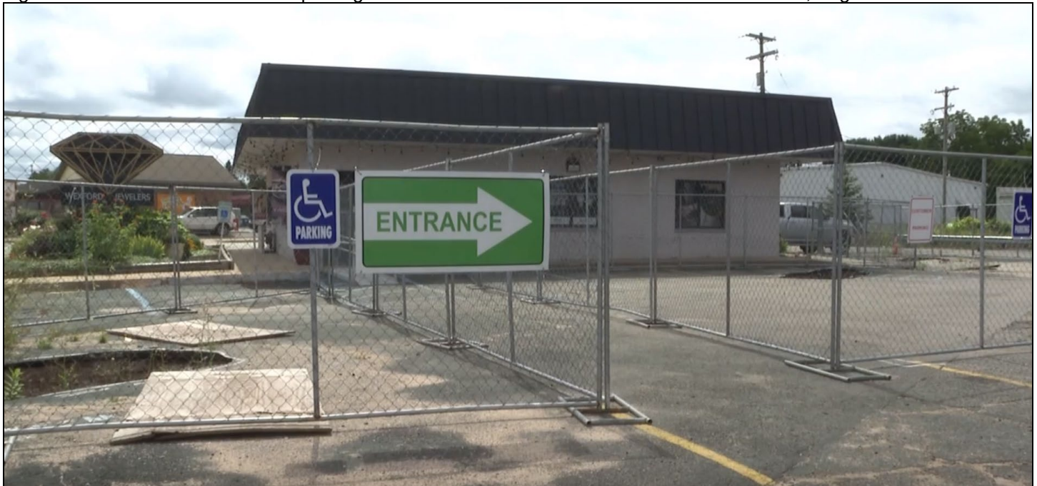
Figure 28. Fenced-off areas of the parking lot of Wexford Jewelers over the Clam River Culvert, August 2023
