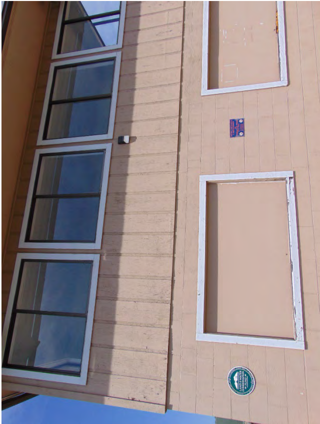
LWCF Recognition plaque on the old concession / restroom building at Herrick Field.
