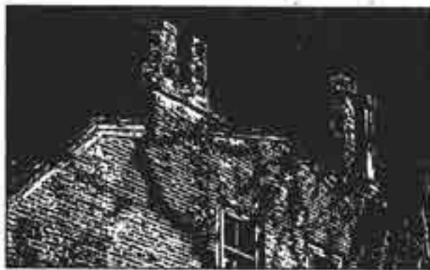
Example of using a longer lens for inaccessible detail. Buttonwood, New Castle vicinity, Delaware.
